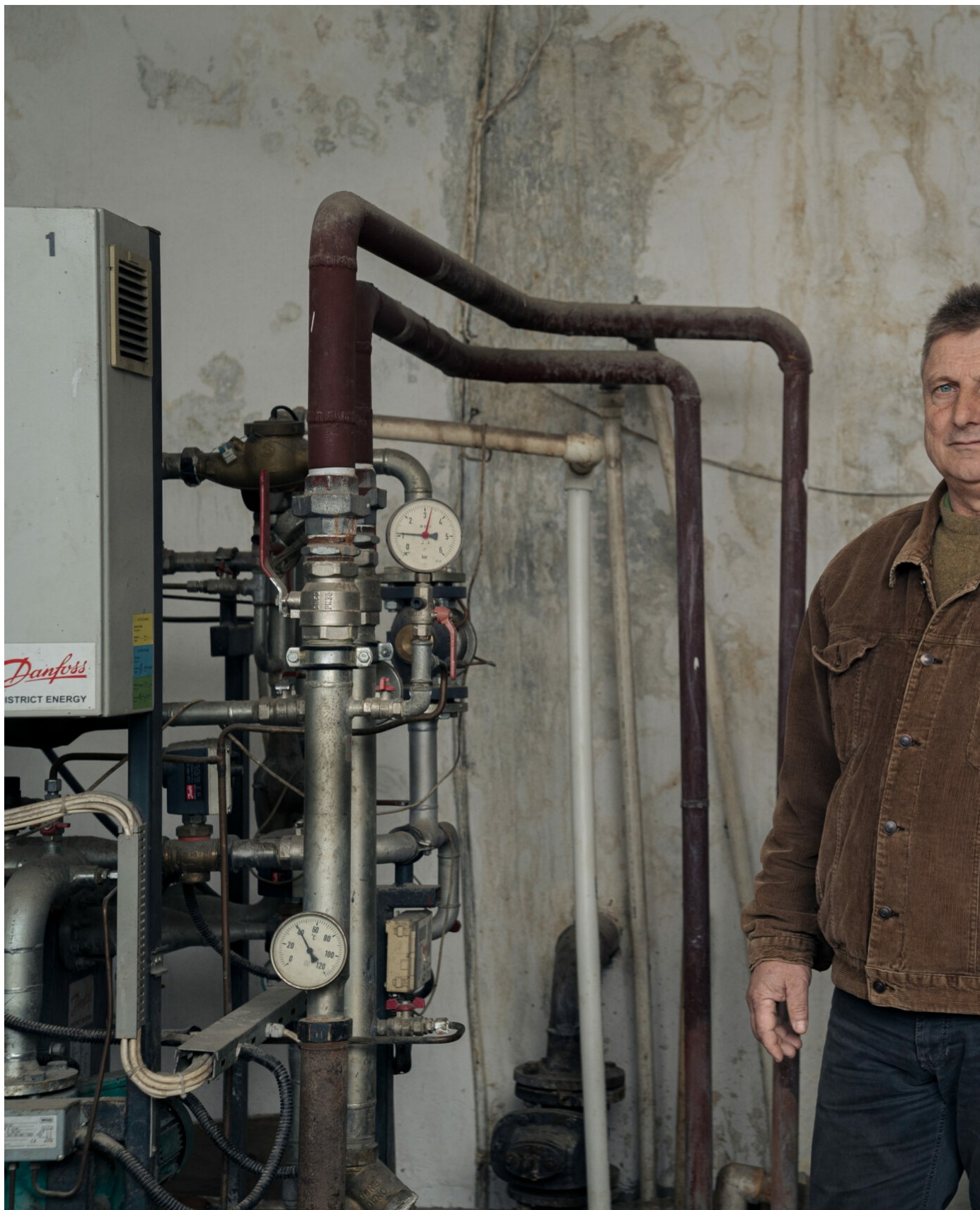
Zamfir Todor, the mayor's advisor in Beiuș, standing next to the thermal module of the geothermal heating system, installed where the old oil-fired boilers used to be until the 1990s. ©Francesco Pistilli
